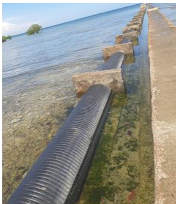
Sea outfall that discharge untreated wastewater to the ocean at Raskazone
