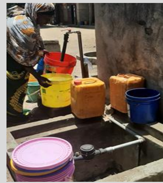
Figure 4-6: Water infrastructure on site which is distributed water taps (Source: Tansheq, 2022)
